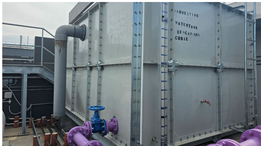
Rooftop rainwater harvesting tank at New DistriPark, Singapore, used to collect and store rainwater for non-potable use.
